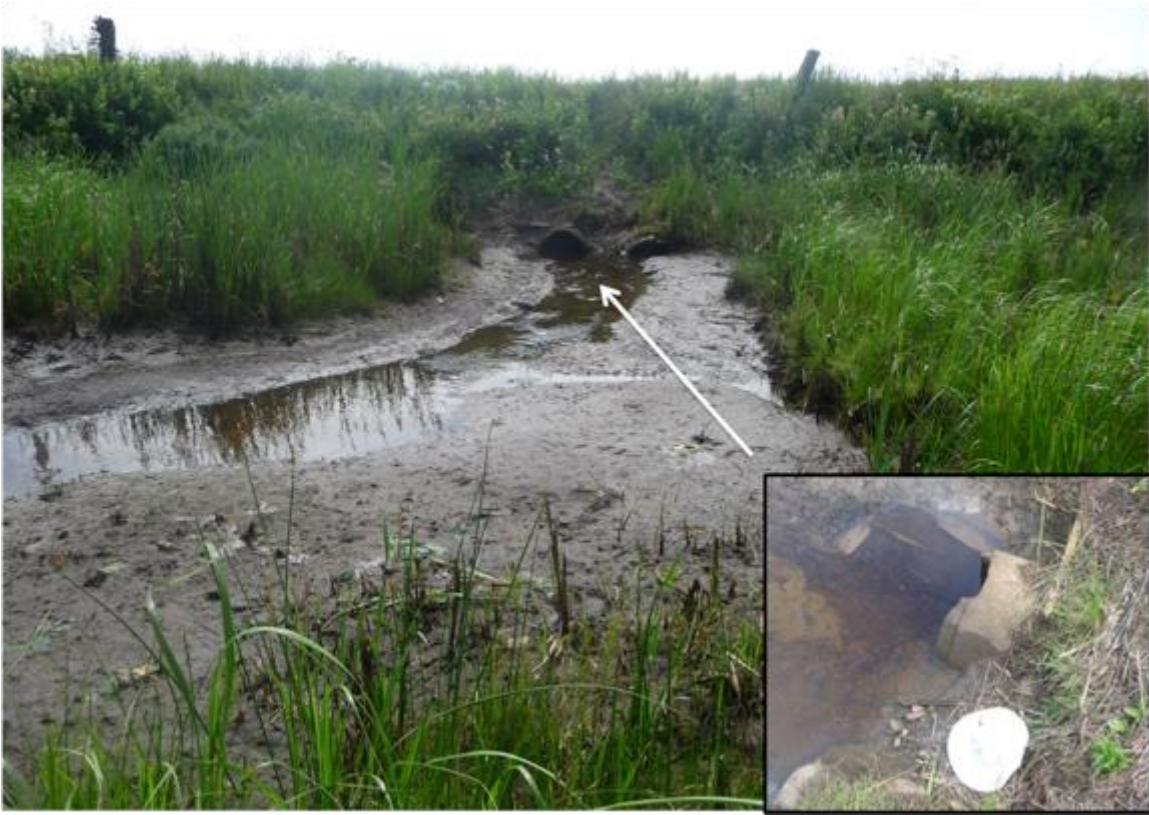
Figure 4 Upstream side of Three Fathom Harbour causeway and culvert shortly after a natural, storm blowout of the buried/plugged culvert. Photographs by T. Bowron, 12/8/11.
