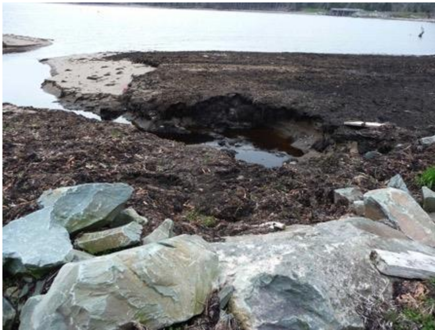
Figure 5 Adjacent beach with accumulated seaweed wrack downstream of the buried culvert. A temporary enlarged channel was created by a rainfall event shortly before the June 25, 2011 photograph.
