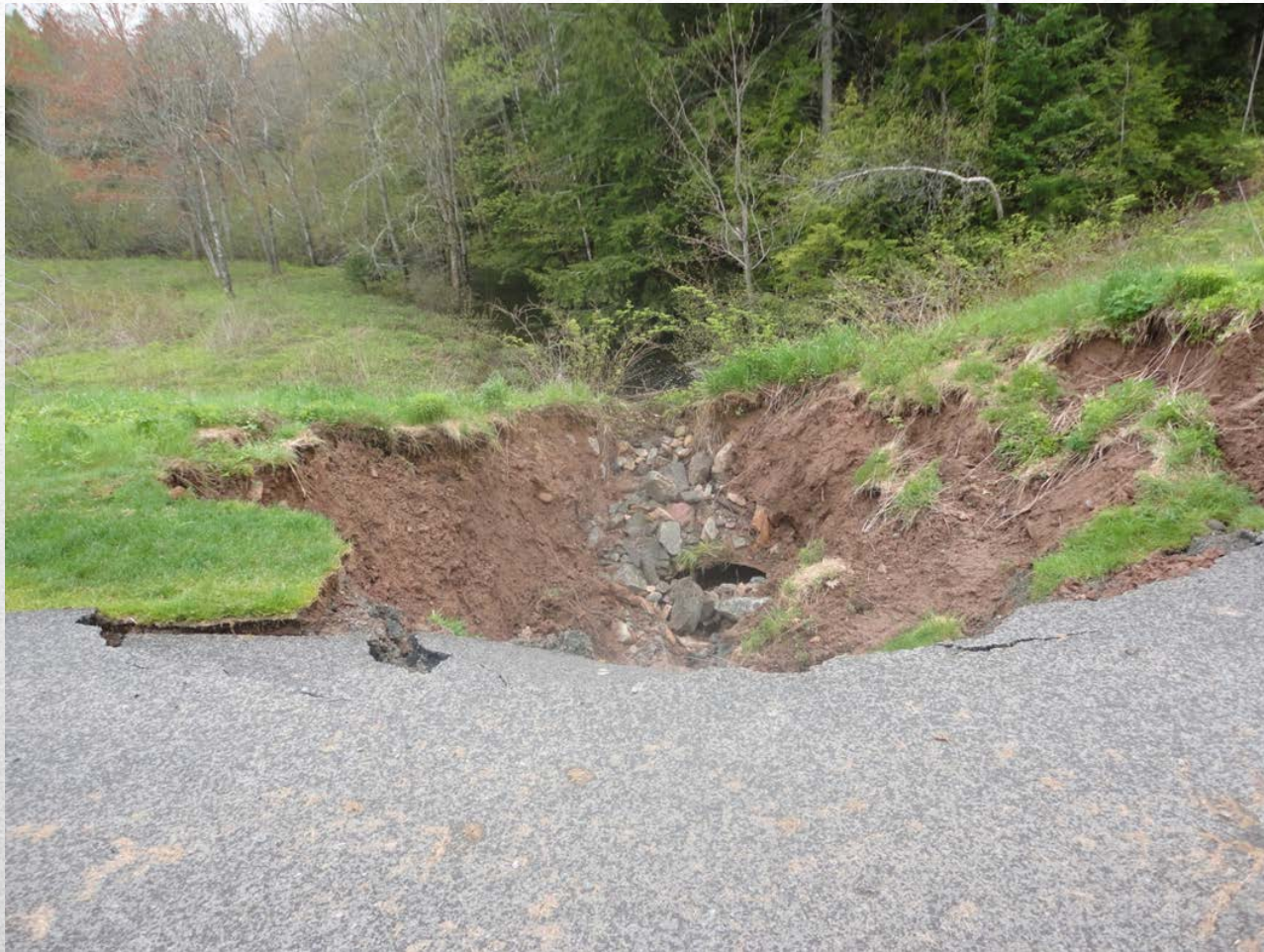
Failed Culvert in 2013
