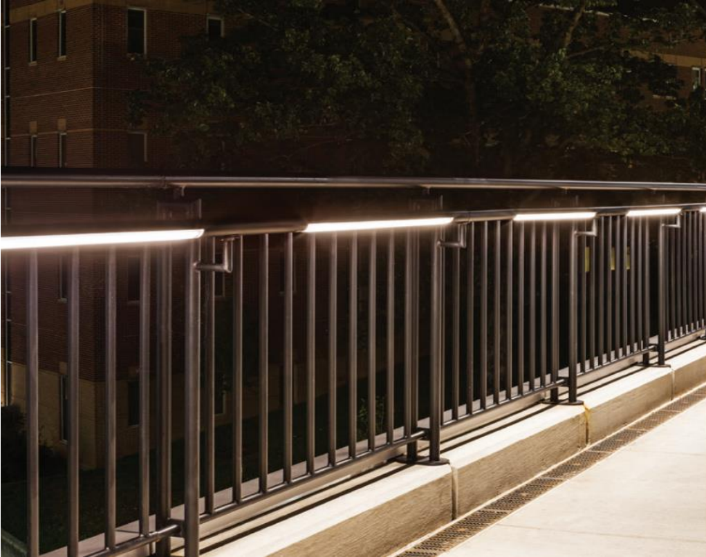
Figure 56: Typical bridge handrail lighting. Source: www.intenselighting.com (n.d.).
