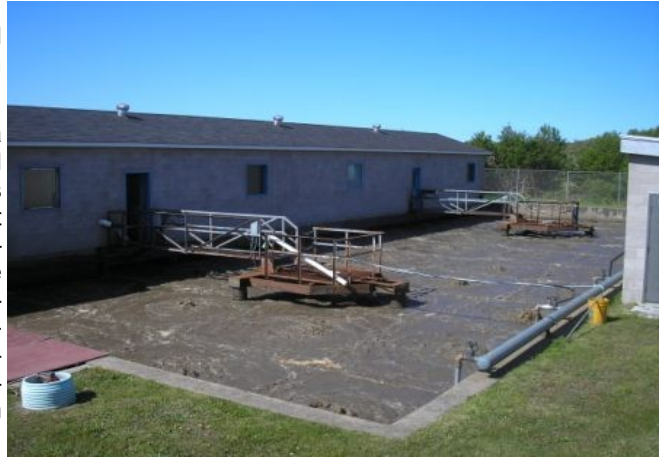
Aeration cell - Digby treatment facility.
