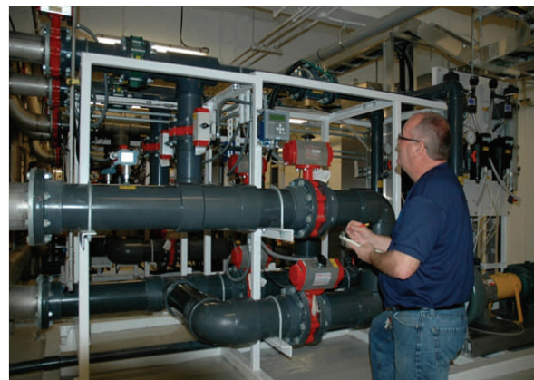
Treatment Plant Operator, Derrick Jessome, monitors the water flow to the primary stage of the UF system.
