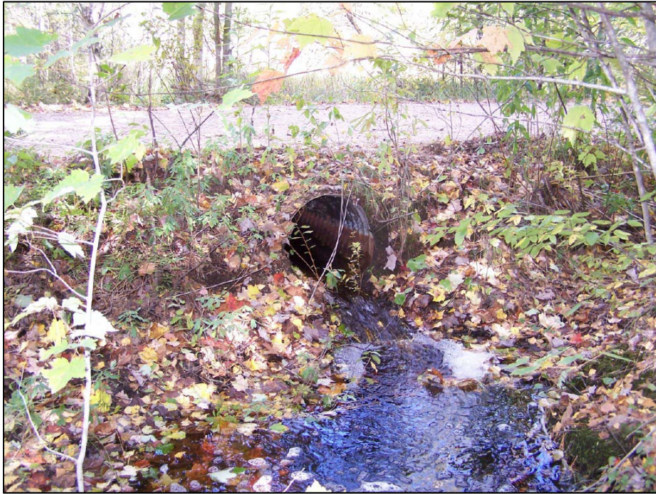
Culvert through railway trail removing excess surface water from the wetland and into a storm drainage system
