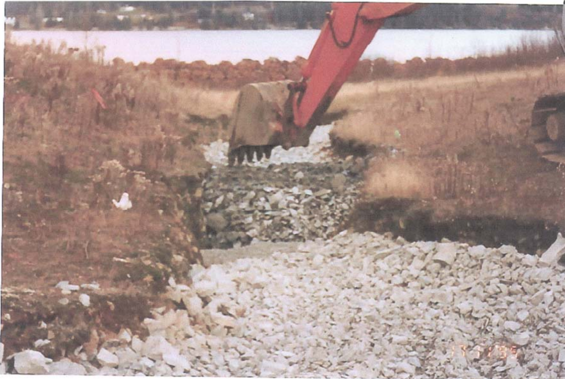
Photo 3: Construction of a bermed ditch along the south side of the Sheet Harbour Industrial Park. Photo taken November 23, 1995.
