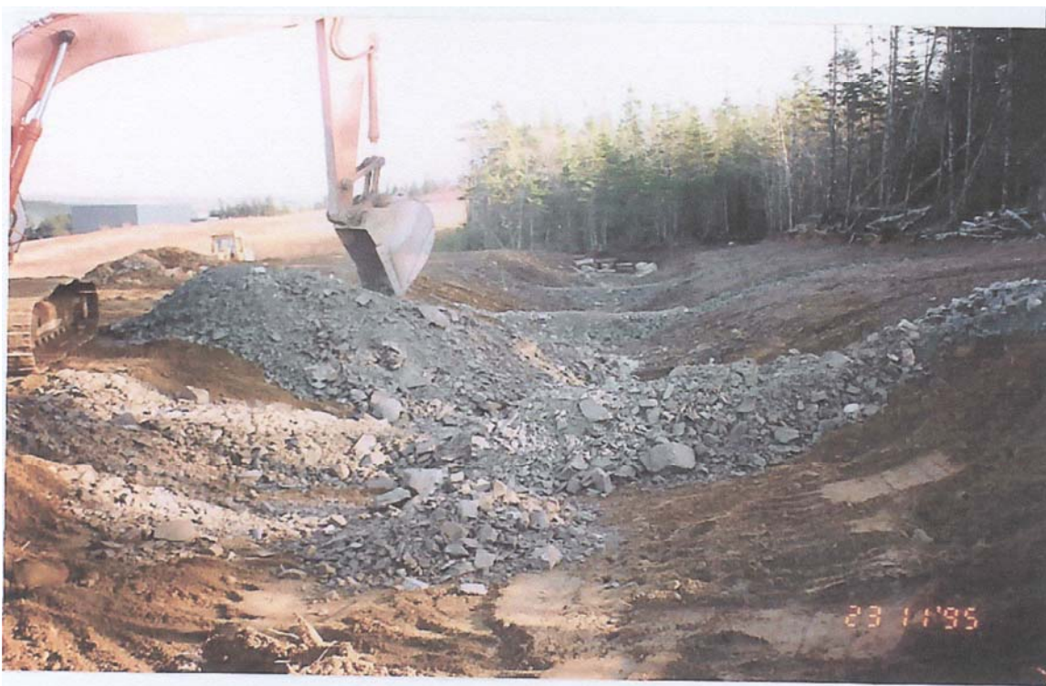
Photo 4: Construction of a ditch on the east side of the Sheet Harbour Industrial Park. Photo taken November 23, 1995.
