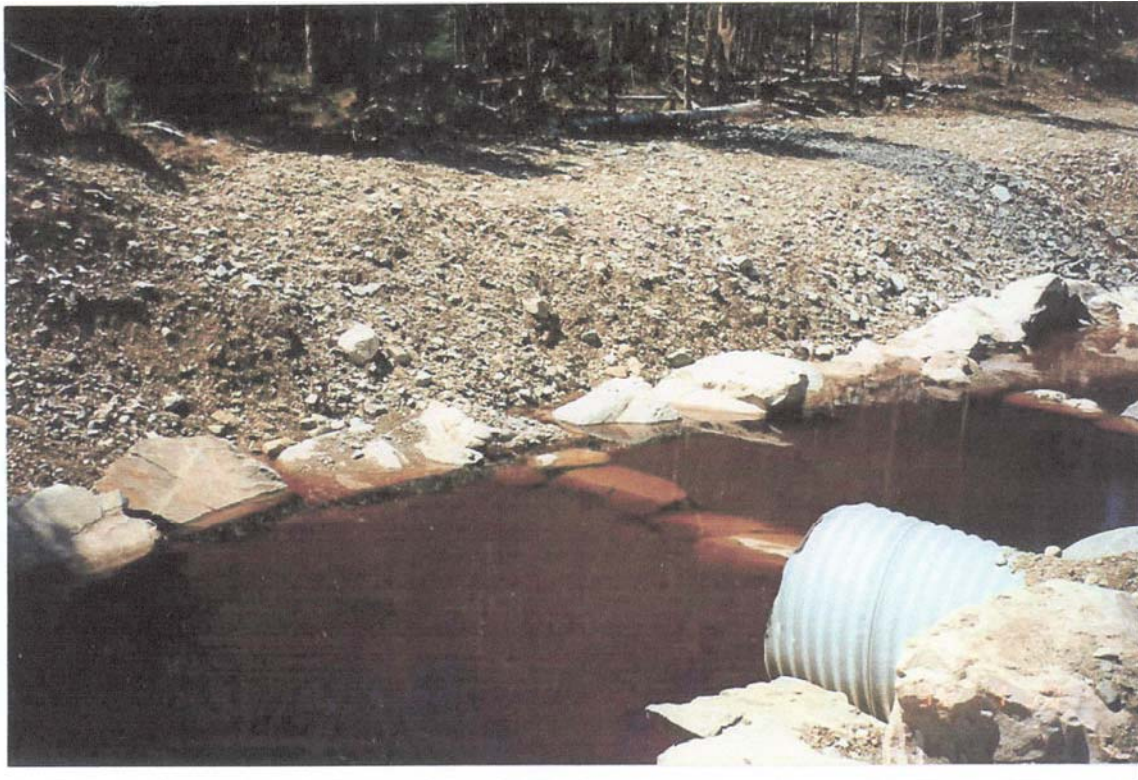
Photo 2: Construction of a french drain on the east side of the Sheet Harbour Industrial Park.
