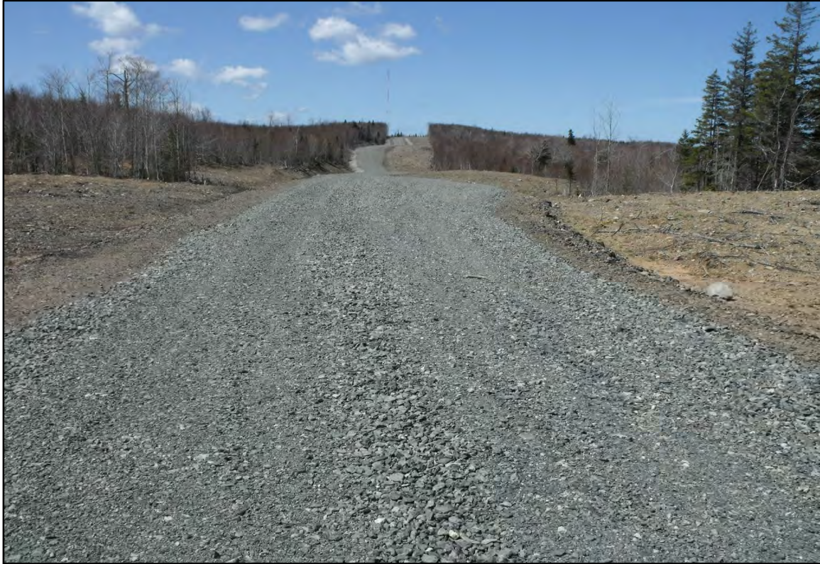
Plate 1: Access road leading southwest up to the MET tower base and pad.
