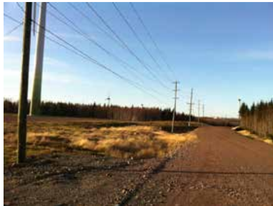
Photo 1. Example of above ground distribution line
