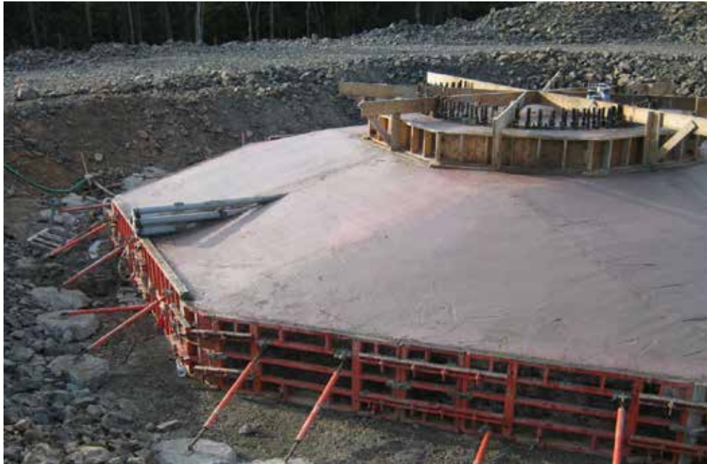
Photo 5. Typical turbine spread footing foundation following concrete pour. Note blasted rock from foundation used on site.
