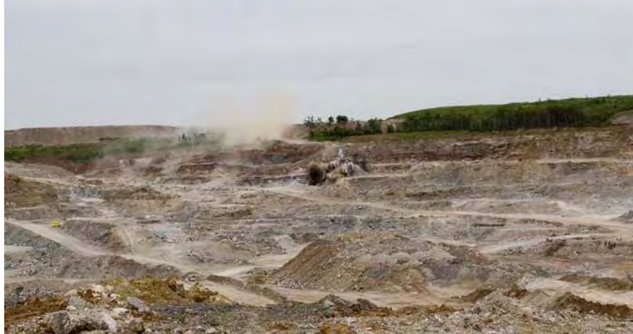
Photo 6.8-3: Second blast site.
