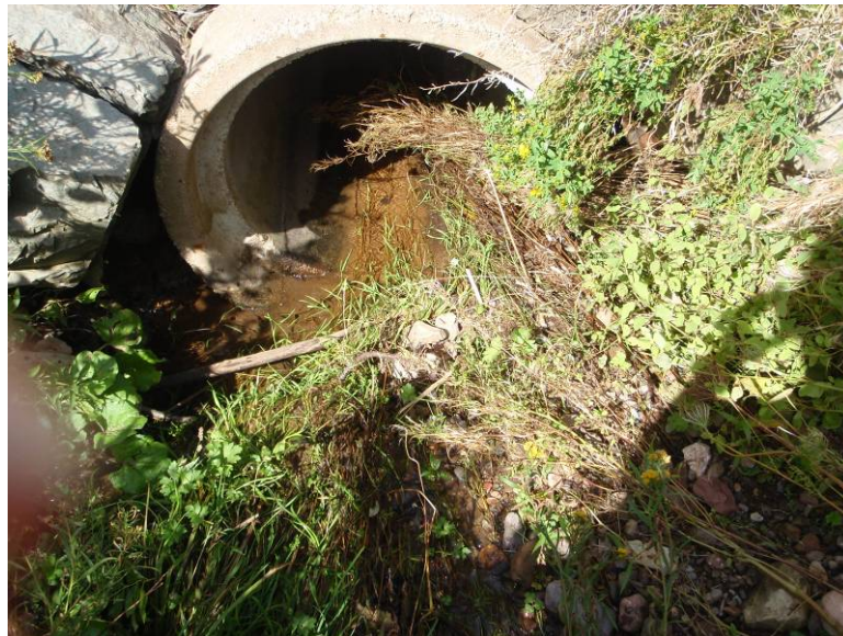
Photo 4.2.5: Flow conditions at SW-11 culvert inlet (September 16, 2008)
