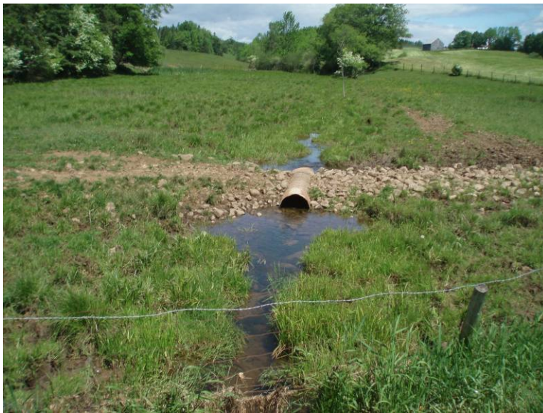
Photo 26: Shaw Brook upstream of Avondale Road, note improperly sized culvert. Cattle have trampled the watercourse banks through this field.
