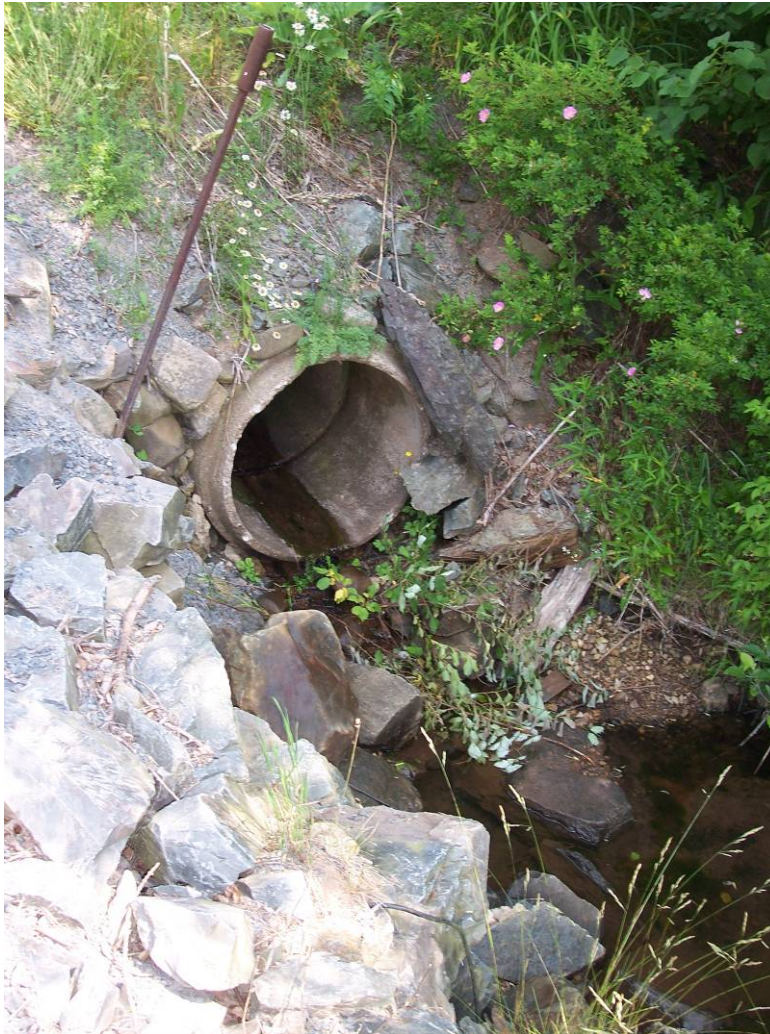
Photo 33: Improperly installed culvert at property entrance off Avondale Road in unnamed tributary.
