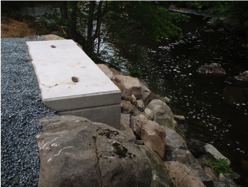
Figure 16: Recently constructed bridge abutment on Herring Cove Brook, immediately downstream of Nickerson's Pond dam. Photo taken September 16, 2014
