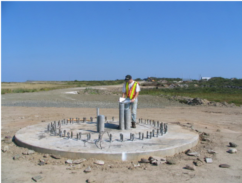
PLATE 4: New turbine base and access road at the 1-B Colliery site in Bridgeport. Facing northeast.
