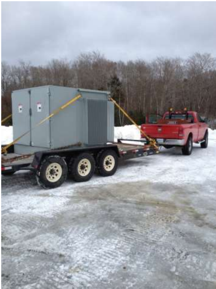
Figure 2.6 Pad mounted step-up transformer to convert 690V from turbines to collector lines
