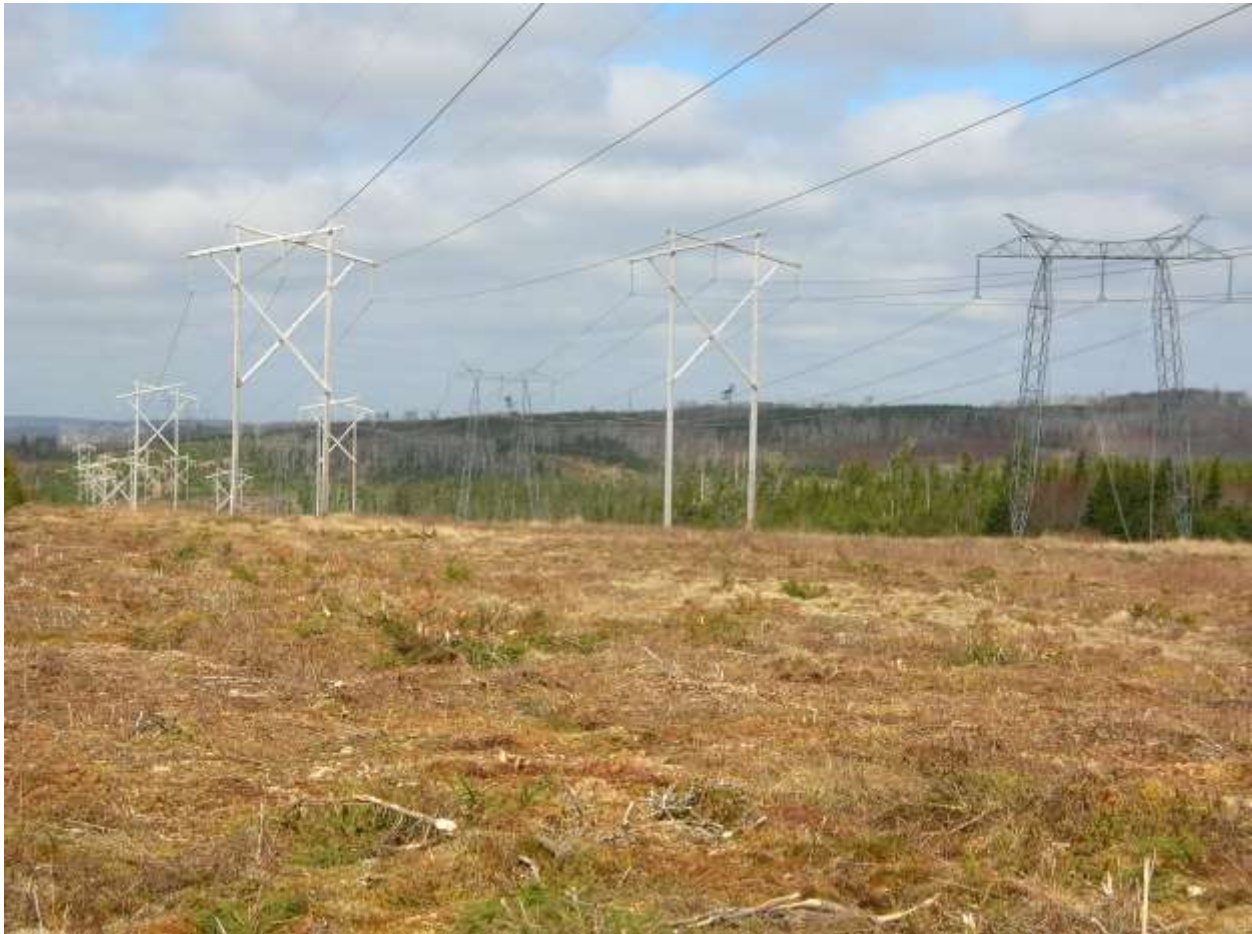
Figure 5.5 Ground cover beneath transmission lines at Kempton
