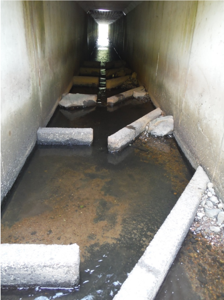
Photo 5.4 WC3b fish passage under Highway 303
