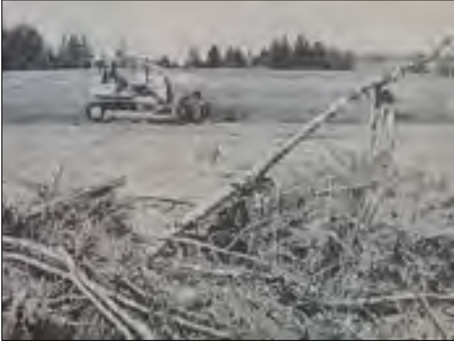
Figure 3-4: A second 1968 image of a bulldozer clearing brush and levelling soil on the former Alms House property. 26
