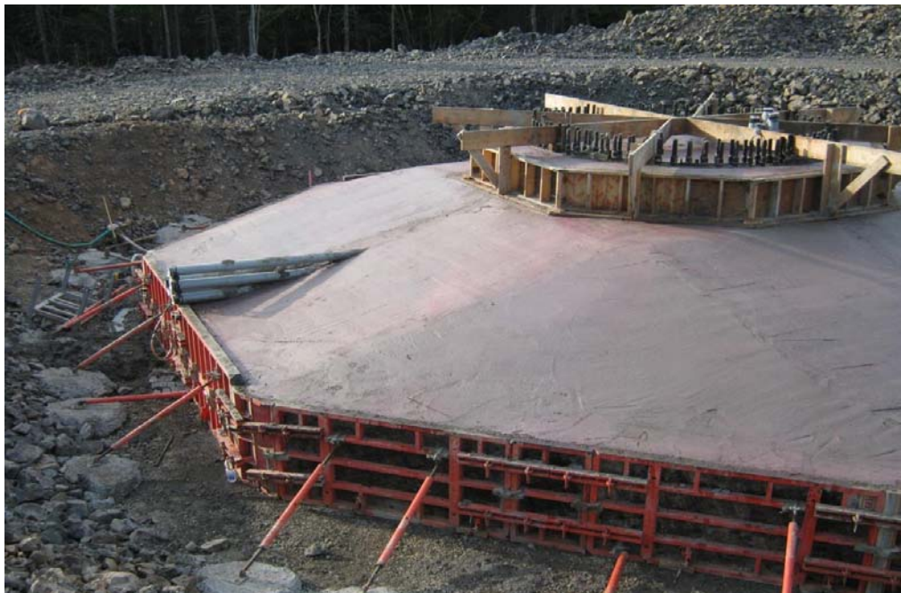
Photo 3. Typical turbine spread footing foundation following concrete pour. Note blasted rock from foundation used on site.
