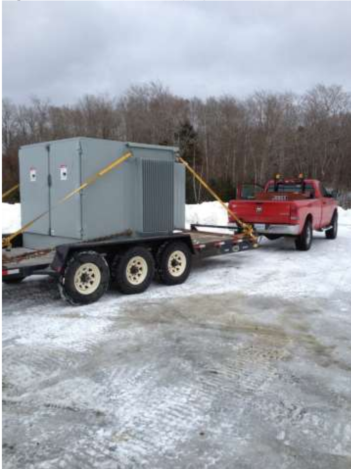
Figure 2.5 Pad mounted step-up transformer to convert 690V from turbines to collector lines.
