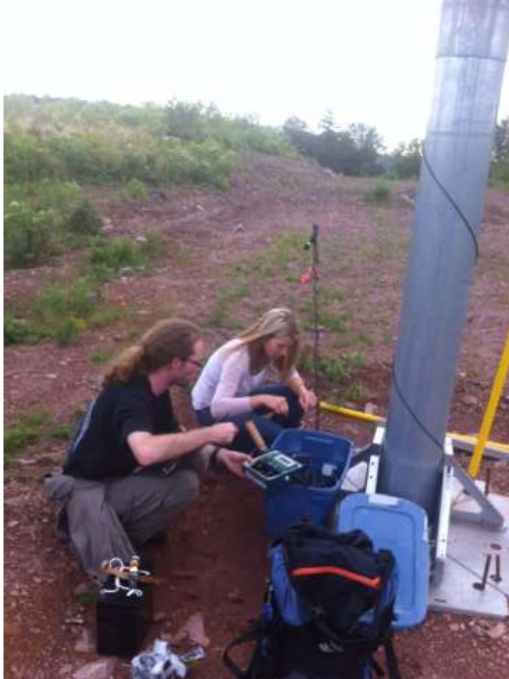
Figure 2.1 Technicians check batteries for bat equipment at the bottom of Greenfield met tower
