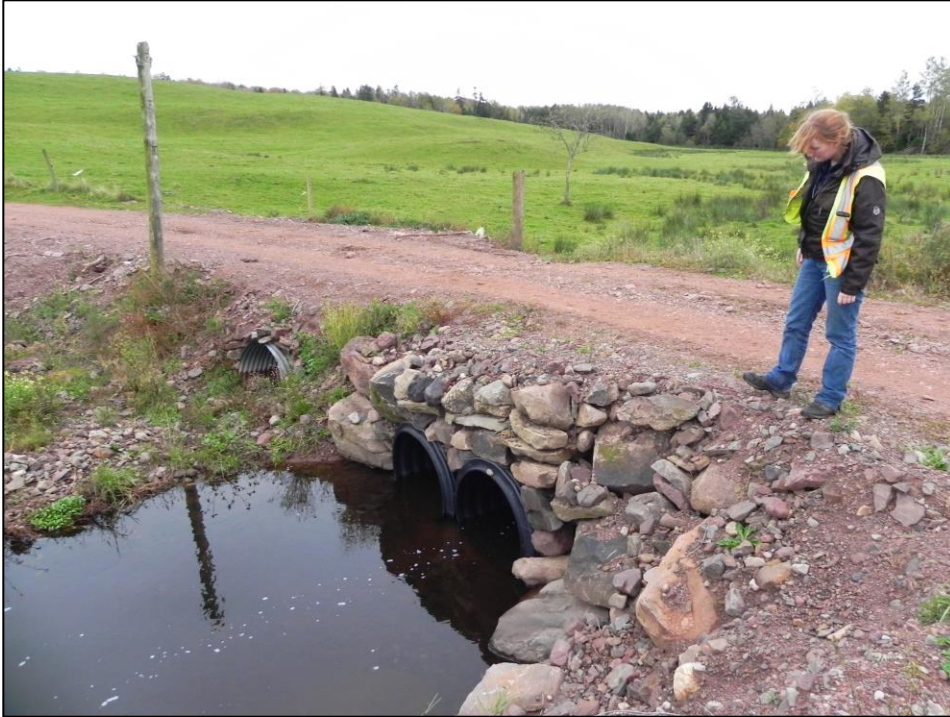
Plate 1: Looking southeast over culverts and watercourse at the beginning of the access road.
