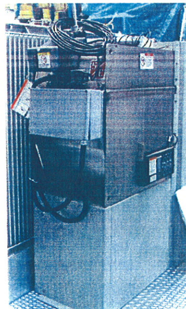
Figure 9: S&C switchgear assembly
