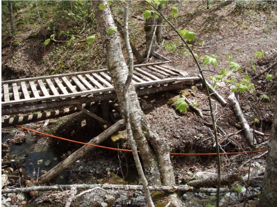
Photos 1c: Existing Bridge on the MacLean's Sugarbush Road Showing Deteriorated Condition
