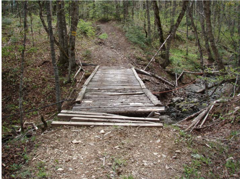
Photos 1a: Existing Bridge on the MacLean's Sugarbush Road Showing Deteriorated Condition
