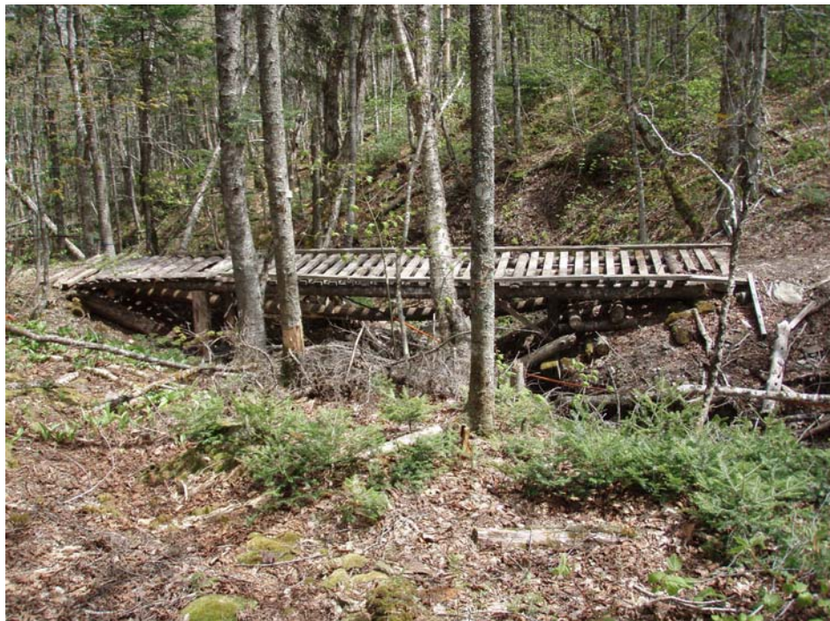
Photos 1b: Existing Bridge on the MacLean's Sugarbush Road Showing Deteriorated Condition
