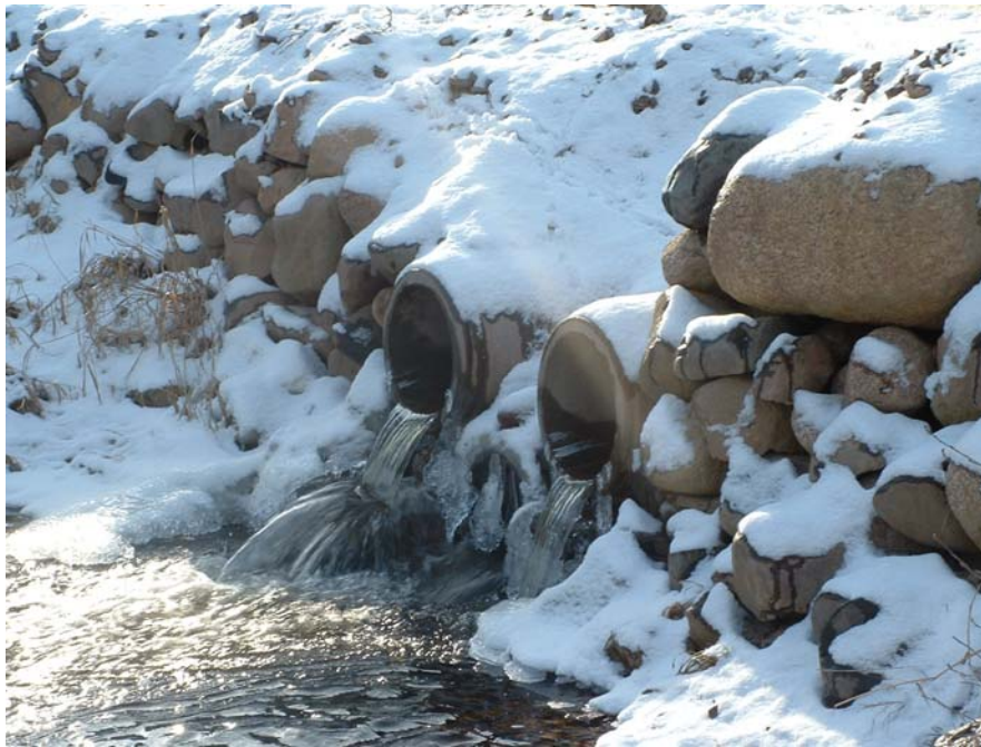
Figure 8: Culvert on pit access road (see: Site C, Fig. 1a). 5 Culverts are used, 2 of which are above the level of the pond and may impose an impediment to fish migration. Water sample BR-2 was taken at this site.
