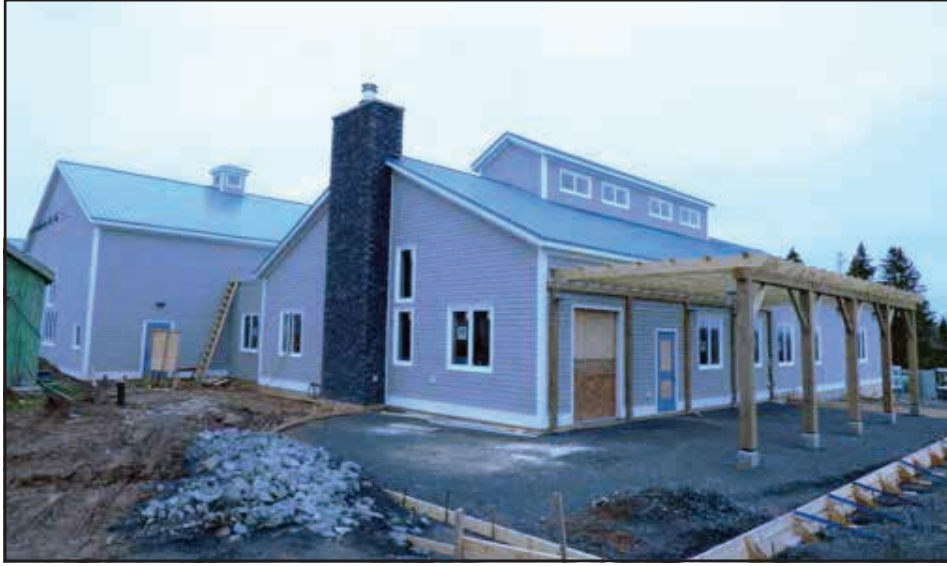
SOMETHING'S BREWING: The soon-to-be completed Authentic Seacoast craft distillery and brewery on Ferry Lane, Guysborough. Contributed Photo
