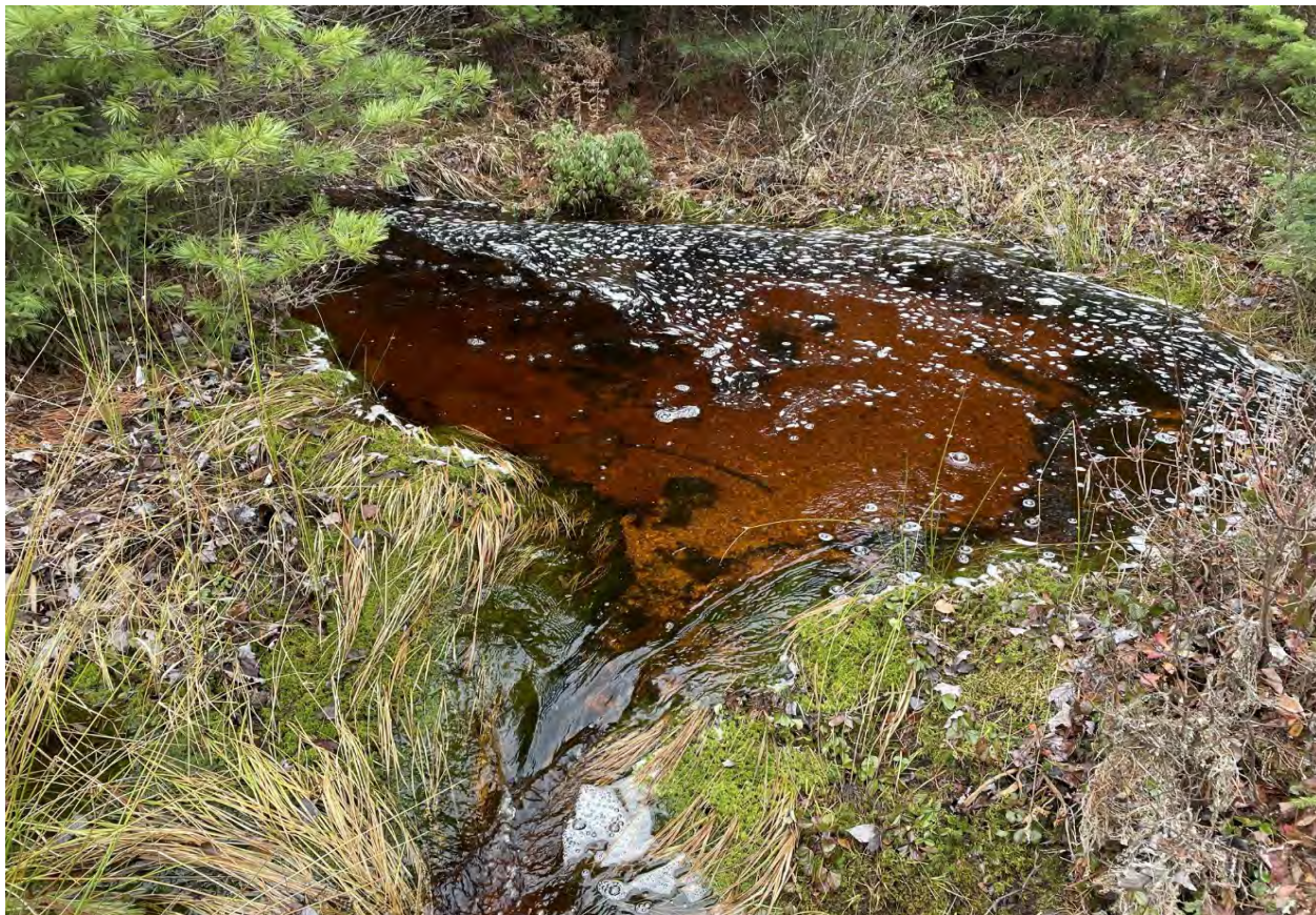
Photo 3: Blocked culvert near road, causing washout
