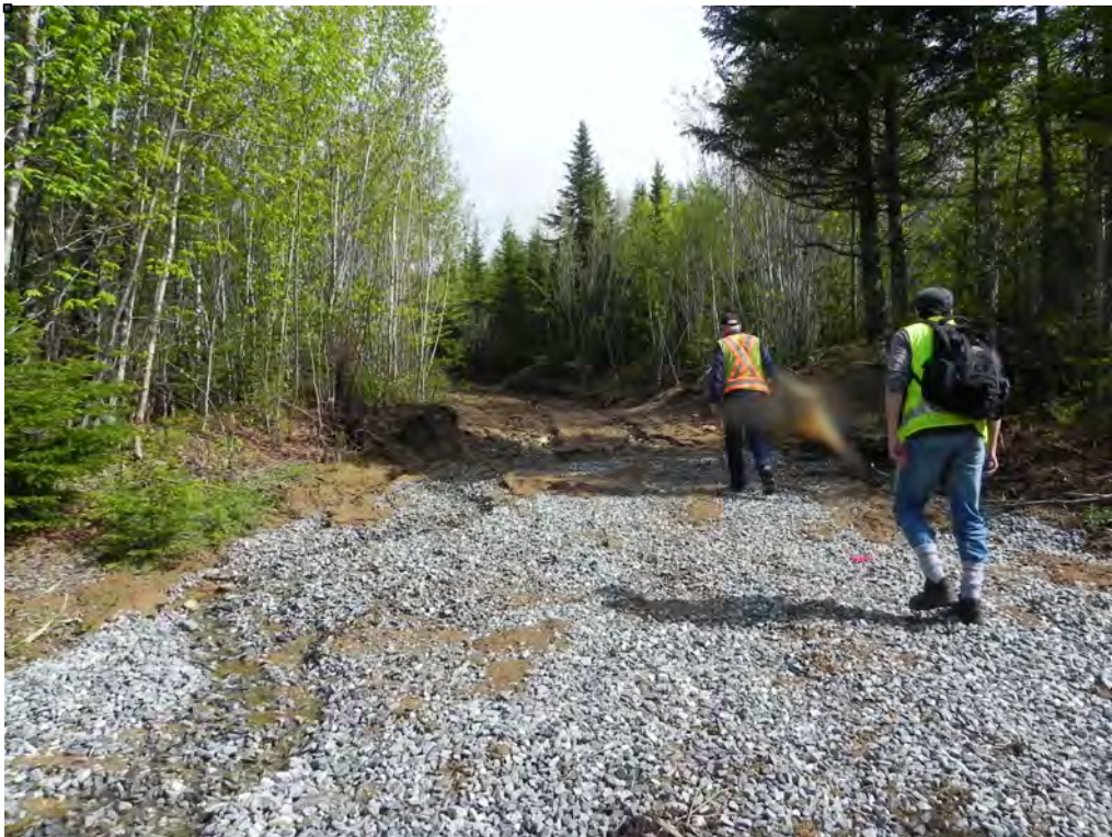
Plate 2: The access road transition from gravel surface to dirt surface. Looking northeast.
