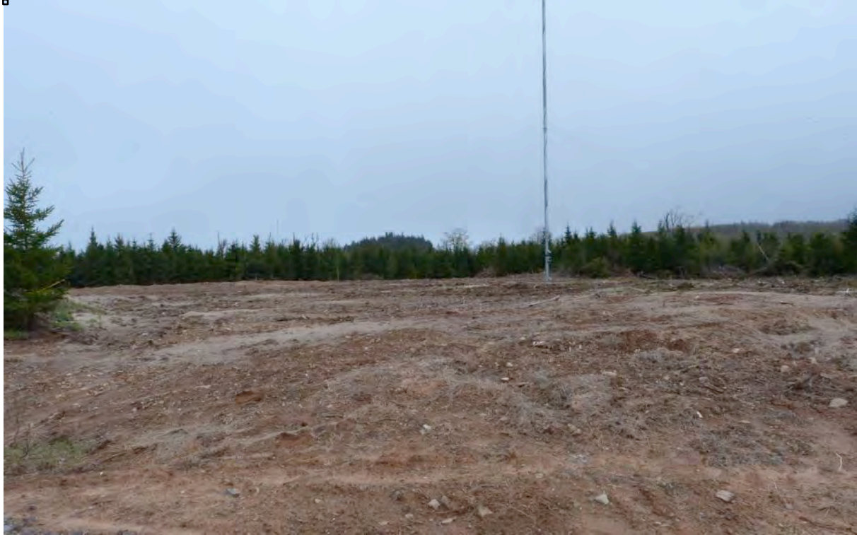
Plate 7: Meteorological tower pad at the end of the access road, looking east-northeast.
