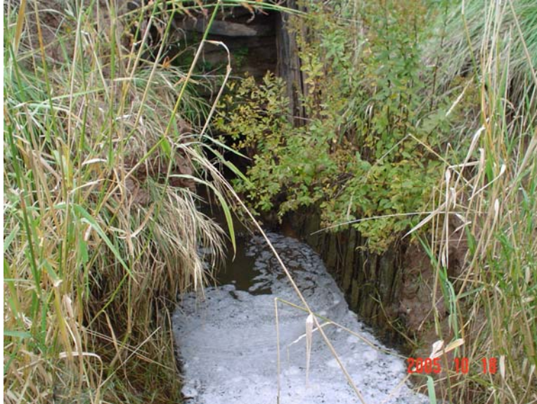
Photo 3: Tributary to the right of LaPlanche River at 977m upstream from bridge, facing culvert, note: white foam in stream
