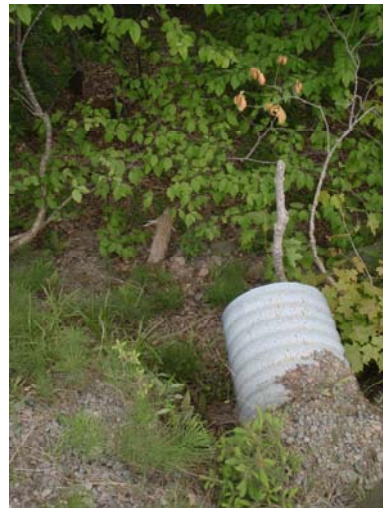
Photo 15: WC-2 – Downstream end of culvert under gravel road, hanging and dry (upstream end buried)
