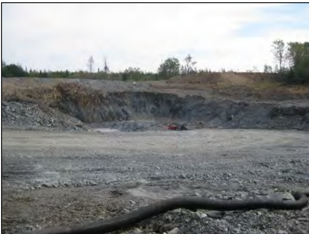
Excavation for Water Discharge to the East of the G&K Tailings Area
