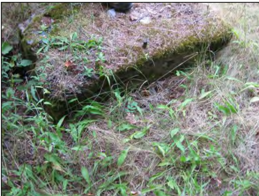
Foundation of a Stamp Mill Located to the South of the G&K Tailings Area Next to the Moose River
