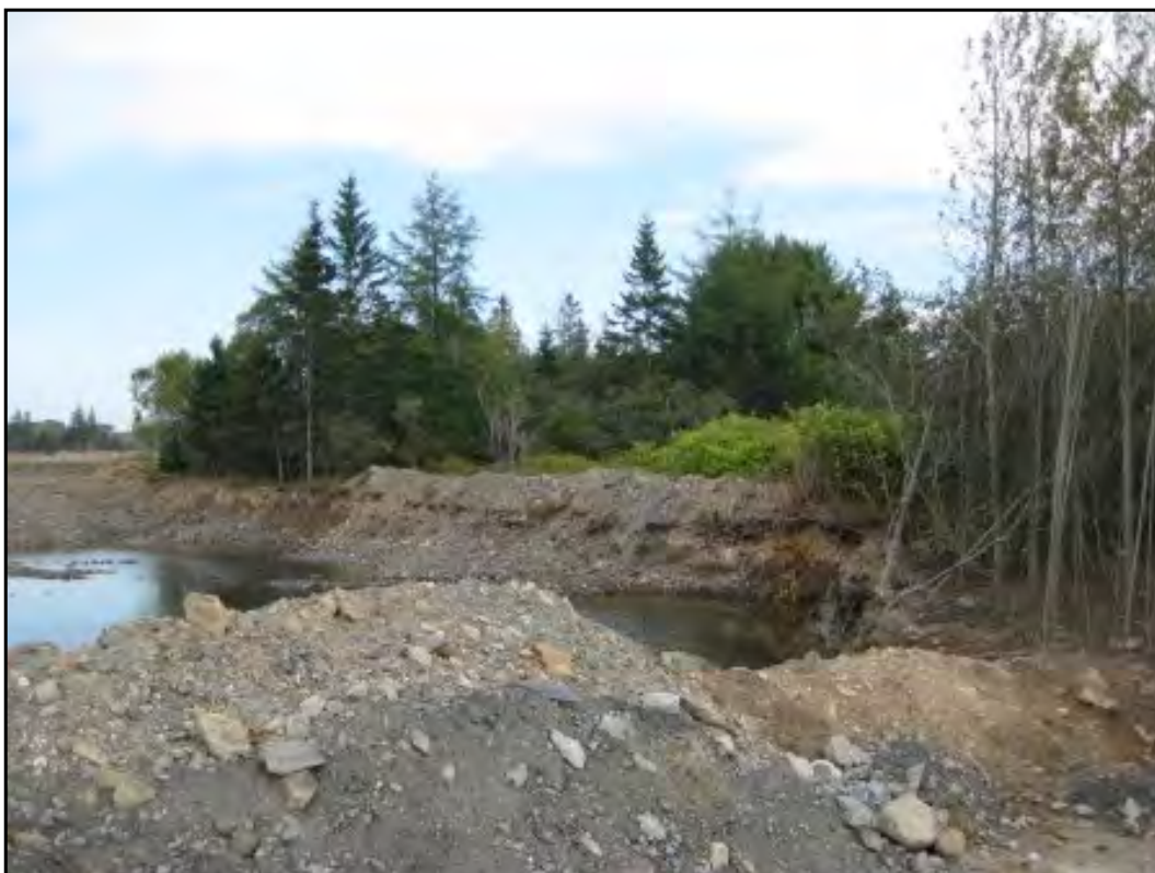
Excavation to the Southwest of the Moose River Tailings Area for Collection of Water
