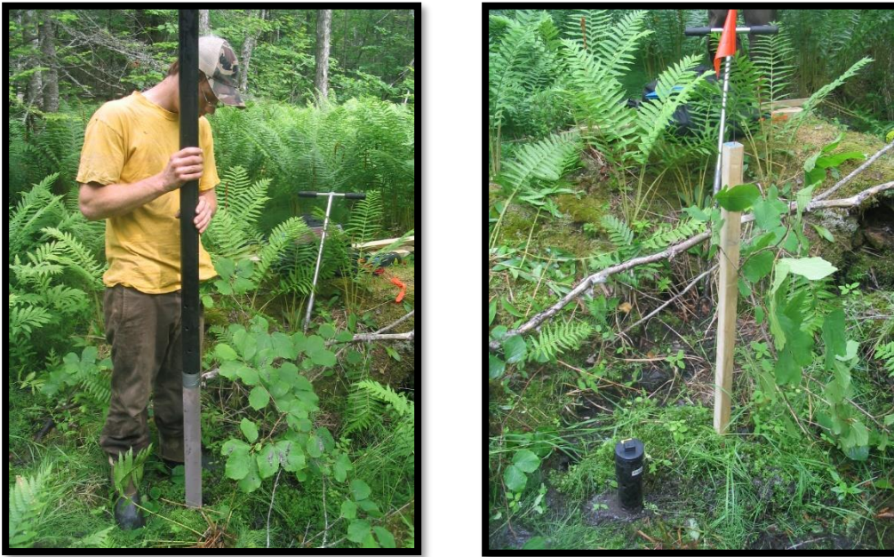
Figure 32: Installation of 2" diameter surface water monitoring wells (l), and a completed and capped monitoring well (r) at Wetland 1.
