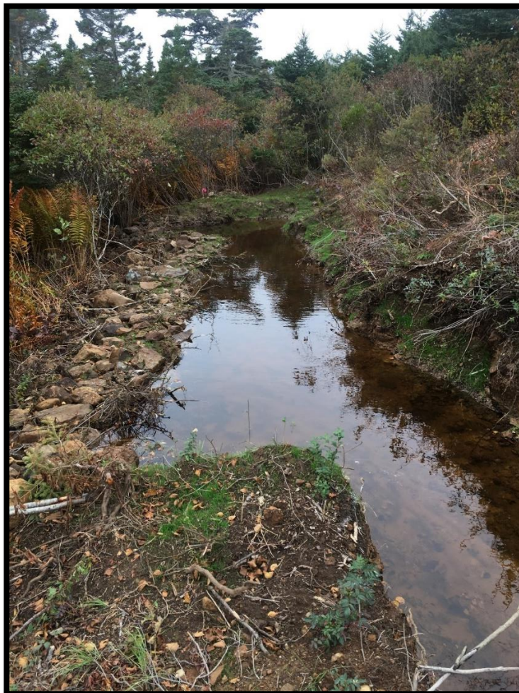
Figure 8: An example of a recently constructed "seep away" structure used to restore a concentrated ditch flow to a more diffuse surface sheet flow at a wetland restoration project on Brier Island, Nova Scotia.
