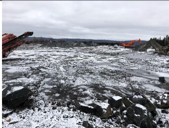
Photo 4: Existing stockpile/Crusher area on the valley floor looking southward from northern extent and the designated crushing area. Temporary asphalt plant designated area is by the excavator in the distance, and weigh scales are image left of the stockpiles located in the image center.
