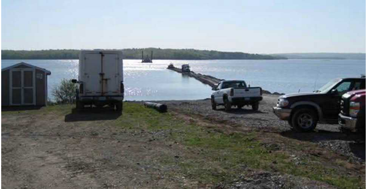
Figure 6. Example of temporary causeway built for HDPE pipeline deployment at the Northern Pulp Mill staging site. Photo from 2009 courtesy of Northern Pulp.
