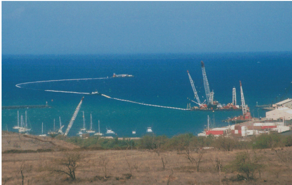
Figure 27. 55” towed deep-water pipeline immediately after assembly and departing for the deployment site.
