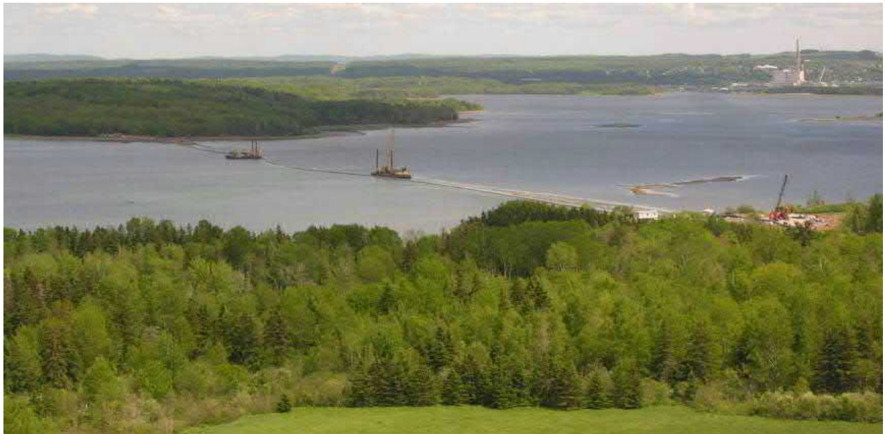
Figure 7. Staged pipeline towed into Pictou Harbor from Northern Pulp Mill, 2009, images courtesy of Northern Pulp.
