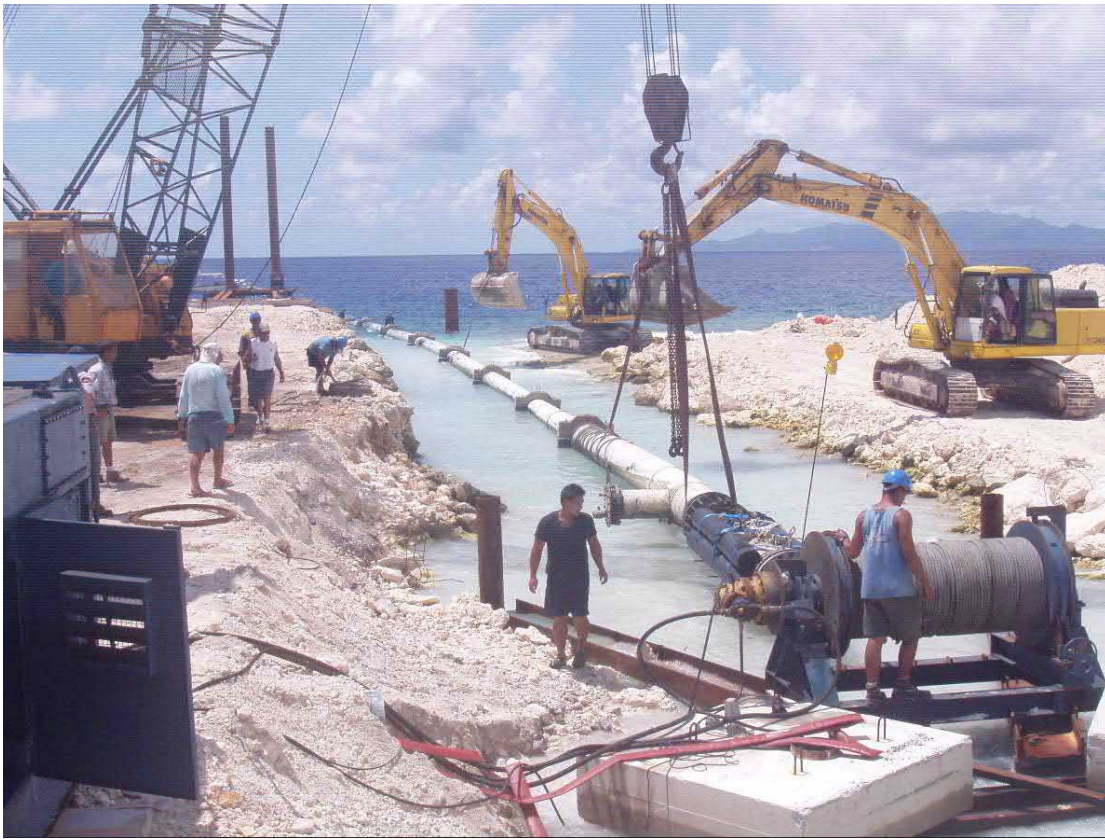
Figure 26. Completed pipe trench with pipe pulled in from offshore by shore winch.
