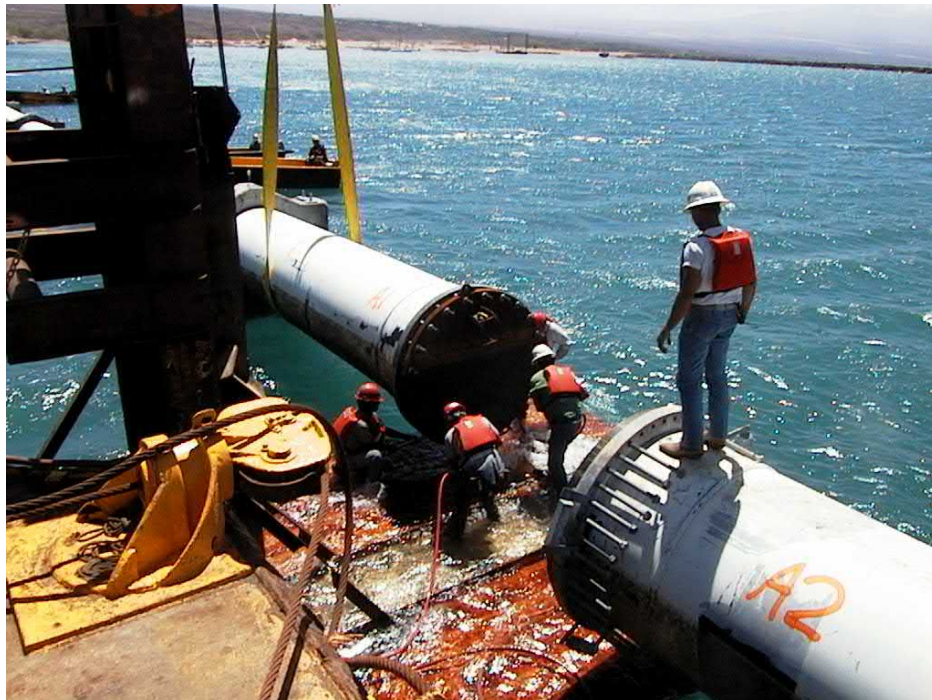
Figure 25. View of elevator platform mounted on a barge – here used for flange connections on 55” pipe in Hawaii 2001.
