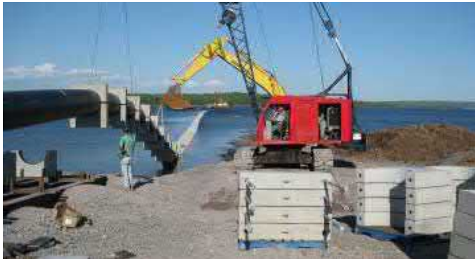
Figure 18. Image of pipeline being pulled into Pictou Harbor, 2009, images courtesy of Northern Pulp.
