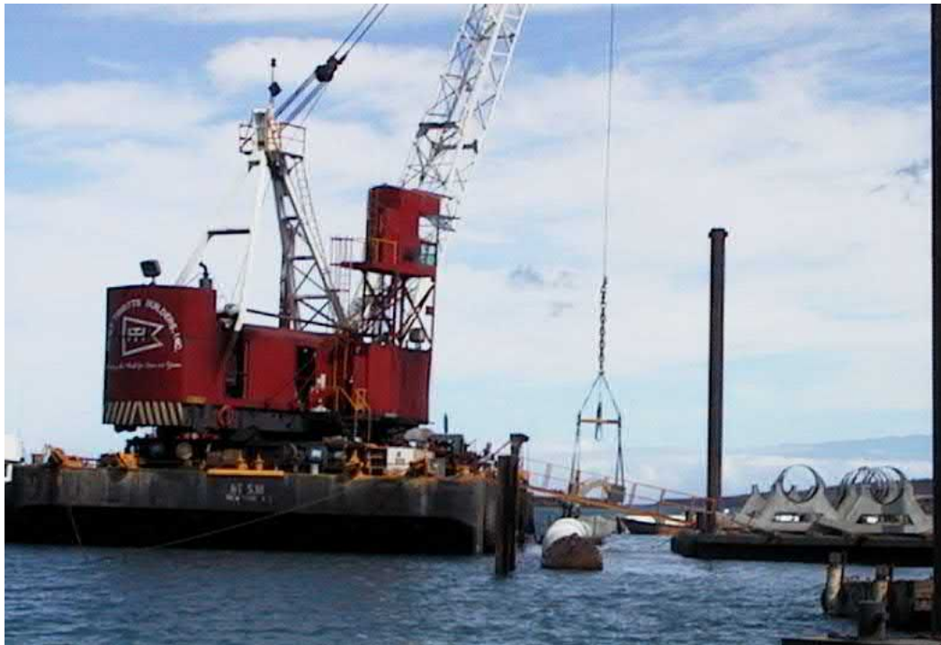
Figure 24. Pipe weights being installed on floating pipeline using a crane barge with an elevator mounted on its side.
