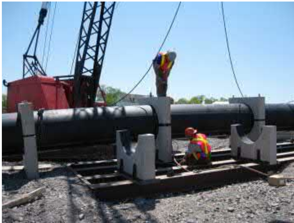
Figure 19. Image of pipe weights being affixed to HDPE pipeline prior to deployment at Pictou Harbor, 2009, images courtesy of Northern Pulp.
