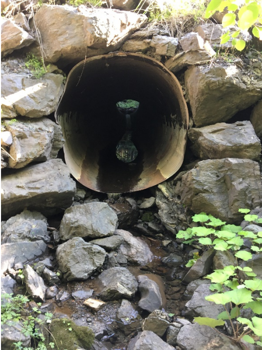
Waypoint 1: Hung culvert beneath Quarry Access Road, looking upstream from culvert outflow. At time of assessment, culvert is impassable to fish and lacks a plunge pool
