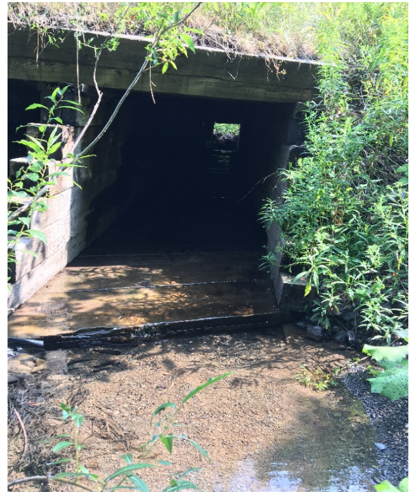
Waypoint 25: Culvert beneath McLellans Mountain Glencoe Road, looking upstream. Wooden, double-box culvert with inflow blocked by debris pile (LWD and gravel/sand).
