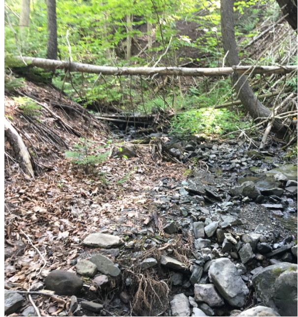
Waypoint 24: Representative of reach downstream of Quarry Access Road Culvert. Water in channel restricted to small pools with maximum water depths of 5 cm. Fish passage/habitat available only during continuous high flow conditions.
