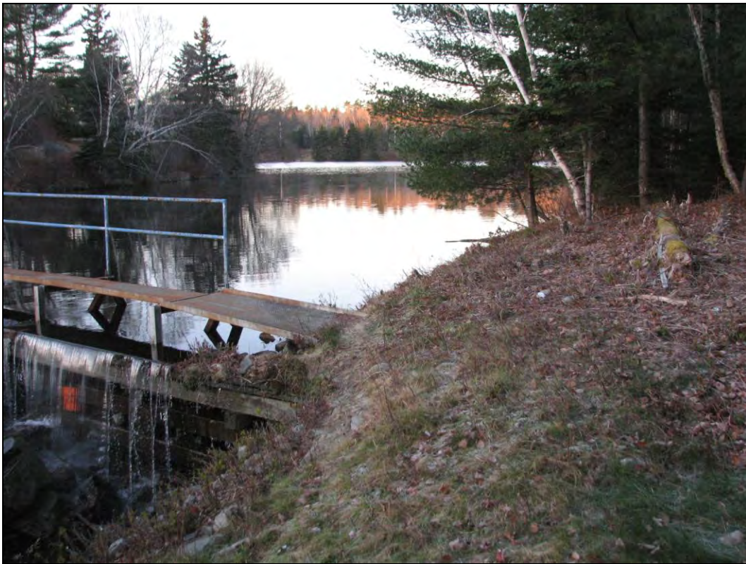
PLATE 1: Lake Major Dam Replacement study area. Existing dam structure and left bank of Lake Major. Facing west. December 5, 2014.
