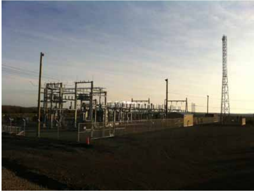
Photo 3. Existing sub-station at Glen Dhu Project
