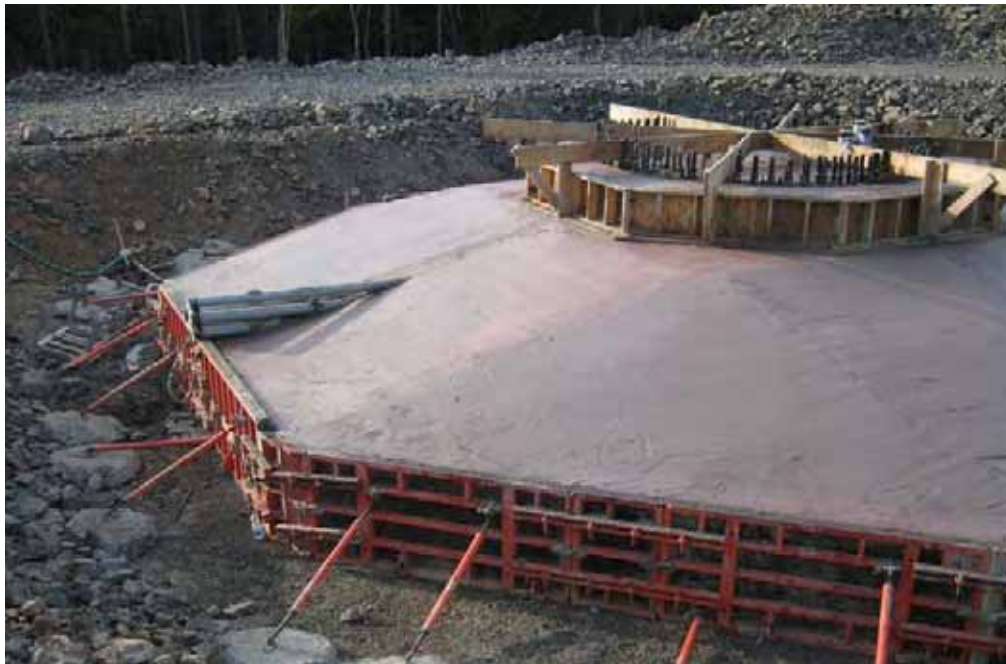
Photo 7. Typical turbine spread footing foundation following concrete pour. Note blasted rock from foundation used on site.
