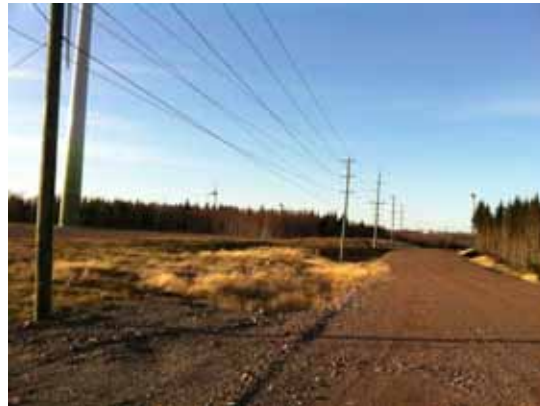
Photo 1. Above ground transmission line on existing Glen Dhu Project.
