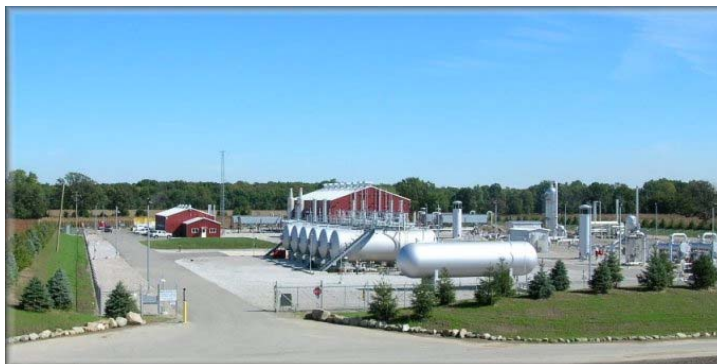
FIGURE 2.4 Example Surface Facility
