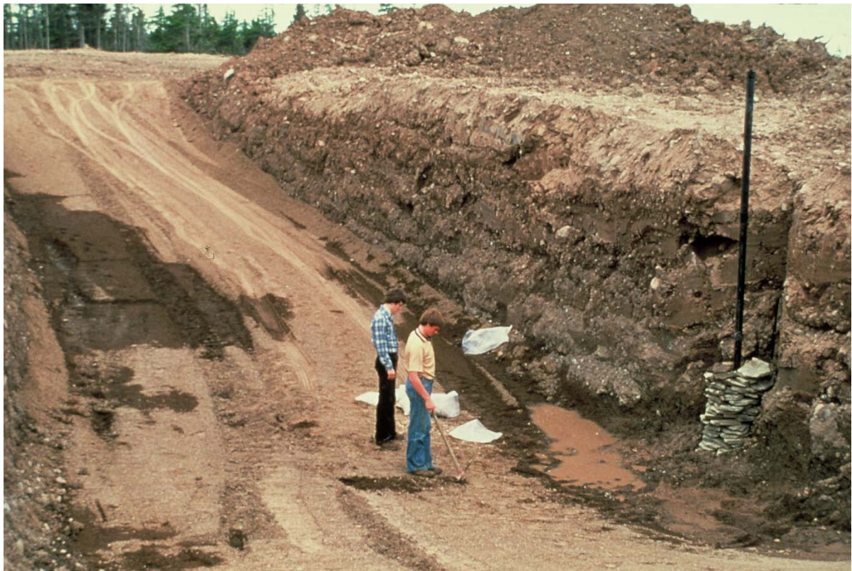
Plate 5-4: Trench 3 ready for disposal with in trench well construction commencing within the east side wall.
