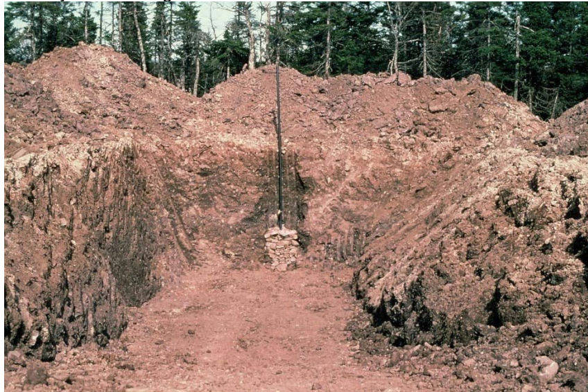
Plate 6-4: Trench 1 ready for waste disposal. Note in-trench monitoring well center background (also present in Plate 6-3).
