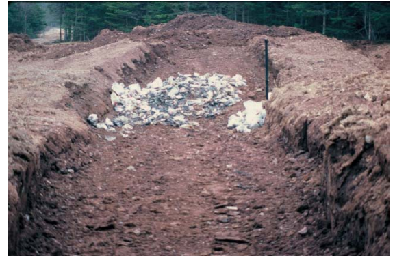
Plate 5-5: Trench 3 disposal with monitoring well construction commencing within the south side wall.
