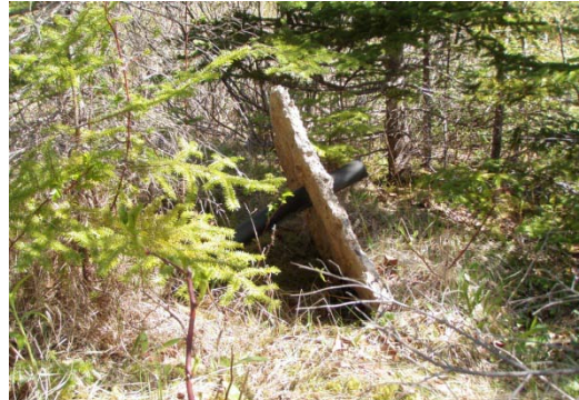
Plate 5-4: Looking east at the damaged in-trench monitoring well downgradient of Trenches 1 and 2.
