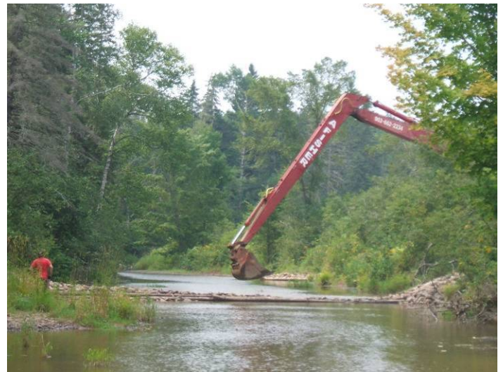
The Cobequid Salmon Assoc. hired a long arm to help add rock to the big deflectors and digger logs installed in Little River, Stewiacke.
