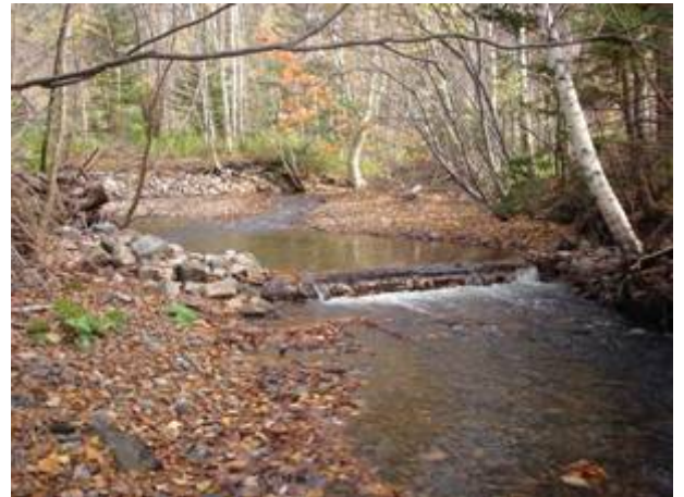
Aucoin's Brook digger log and bank rocking by Cheticamp River Salmon Association
