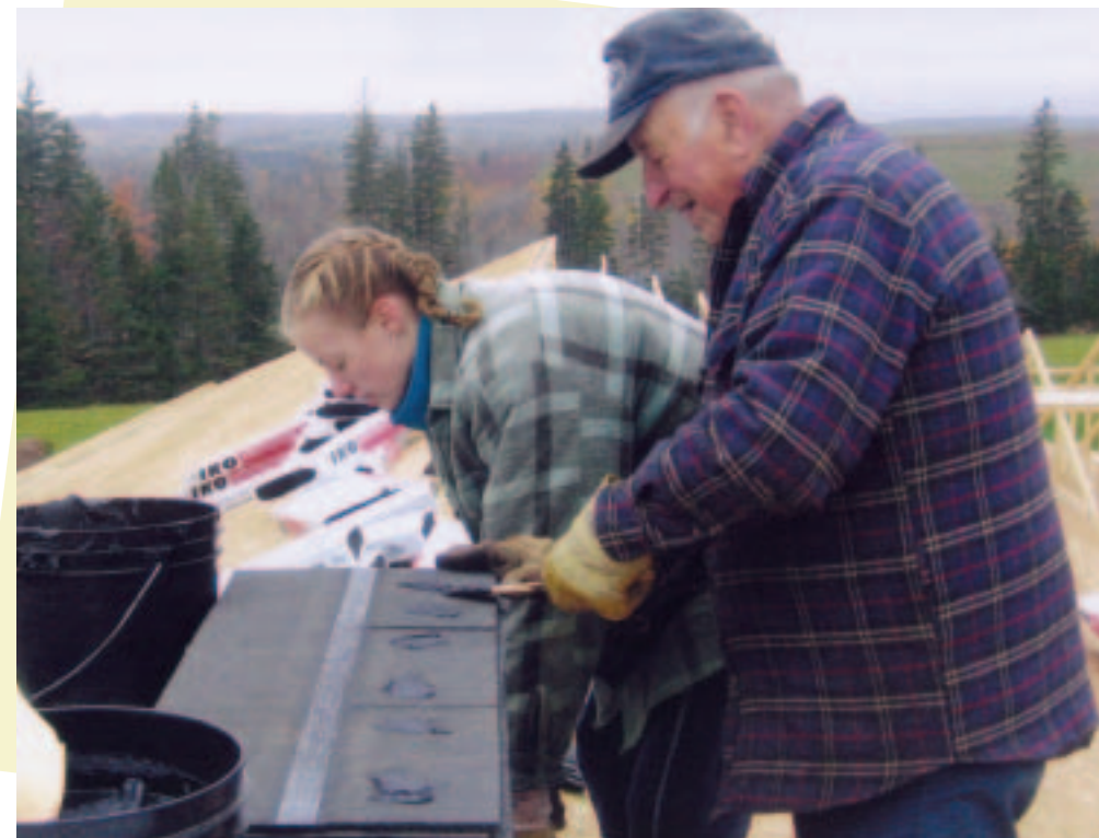
Photo above: Volunteers of all ages lend a hand in creating affordable rental housing for seniors in St. Andrews, Antigonish County.
