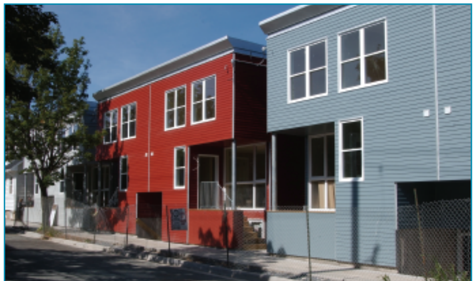
Under the New Home Purchase program , 6 affordable semi-detached housing units were constructed in the north end of Halifax ▶
