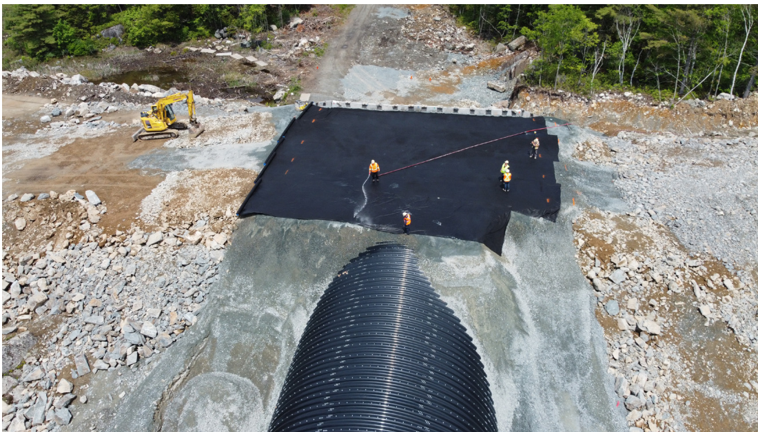
Dexter Construction workers backfill the Pewter Lane arch bridge on Hwy 107 which enables Department of National Defence to access their land on two sides of the highway, via Pewter Lane, which will pass under the highway.
