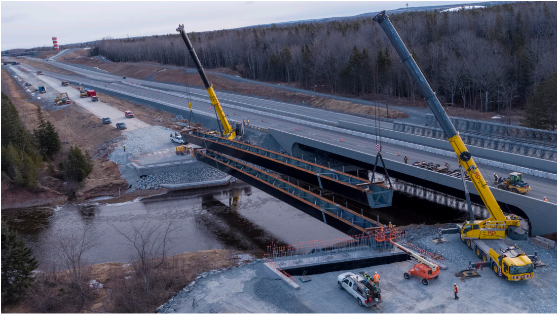
Work this Fall on a bridge over the Nine Mile River on Highway 102
