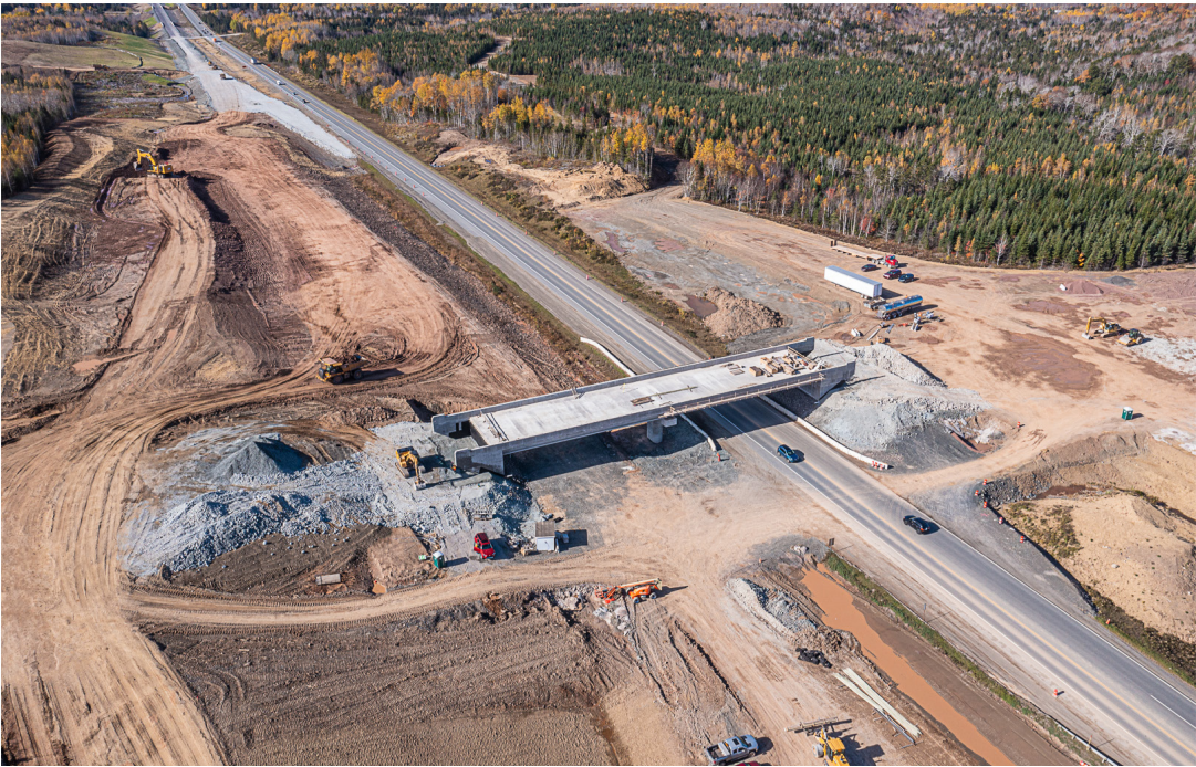
The Barneys River interchange under construction as part of the Highway 104 twinning project.
